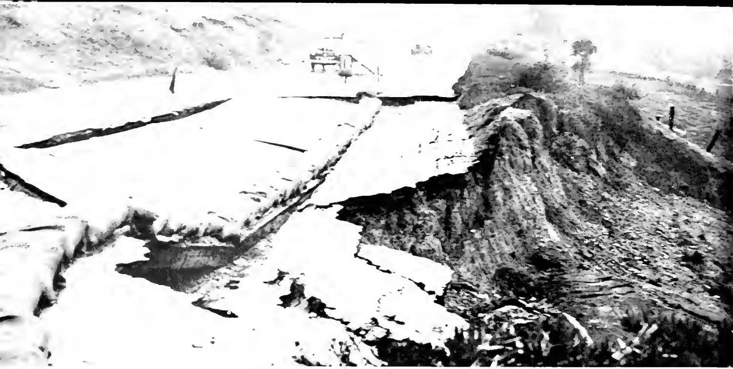
Section of Coast Road (U. S. 101) in Santa Barbara County washed out by flood due to blocked drainage
